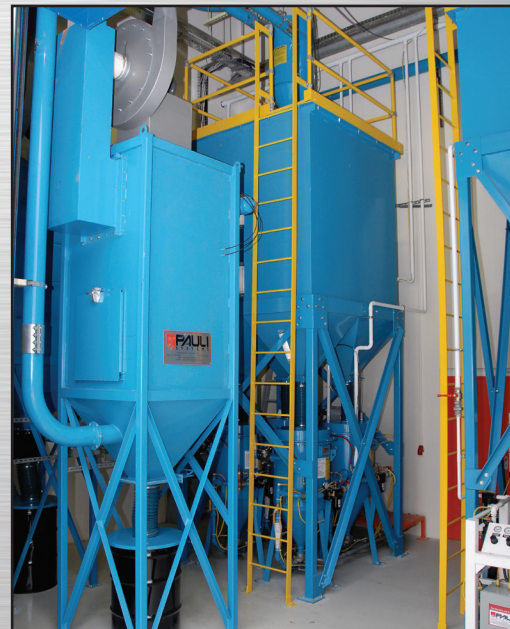
Clean Media Transfer Dust Collector, Clean Media Hopper, Four Stripping Generators.
