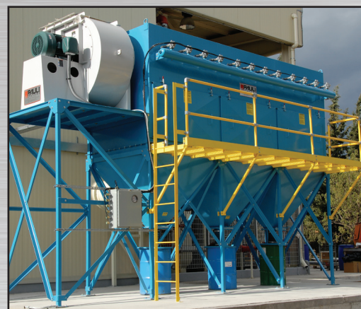
One of Two Dust Collectors Ventilating the Facility.
